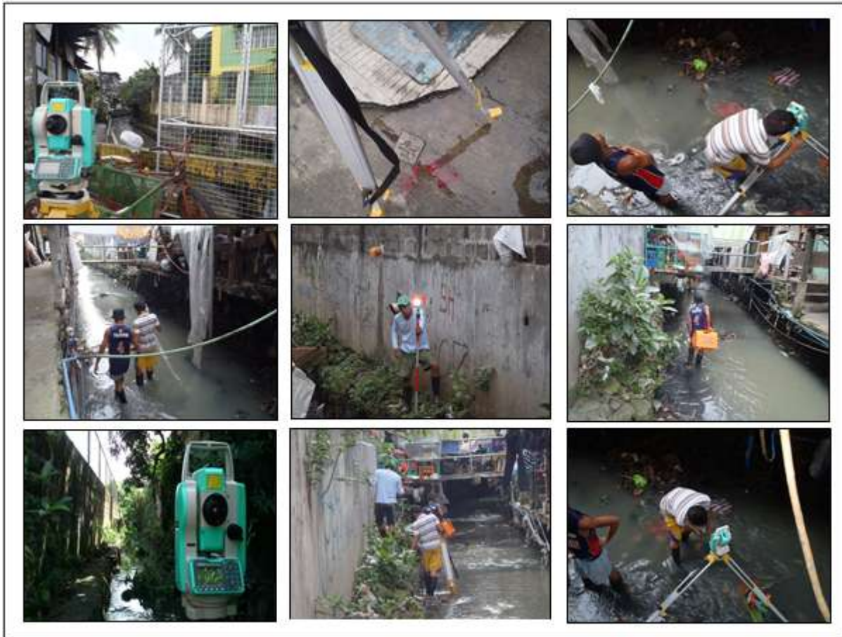
Figure 51. Pictures showing the conduct of profile and cross-section surveys in Kamias Creek which is a tributary of San Juan River.
